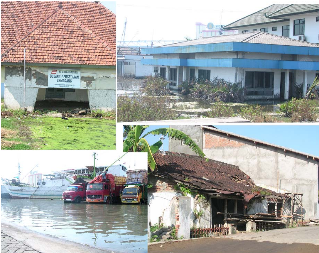
Fig.3. Subsided infrastructures at Semarang coastal city
